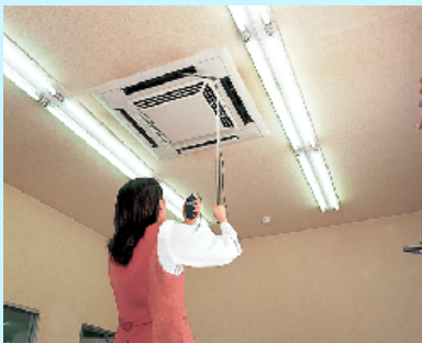
Check airflow rate of air conditioner
