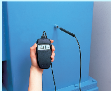
Measuring airflow rate inside duct
